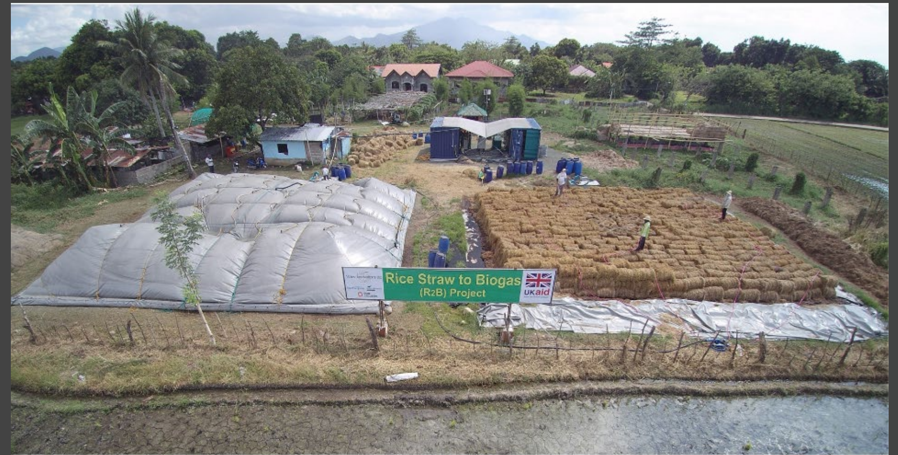
Rice Straw Biogas Facility in the Philippines (Straw Innovations)
